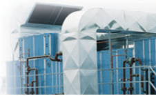
Air Handling Unit
