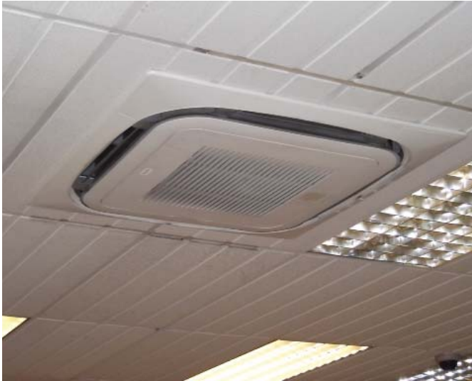
Picture above: Coral betting office self-cleaning cassette after 12 months use
