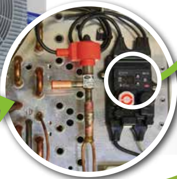
Electronic direct expansion valve and electronic control unit.
